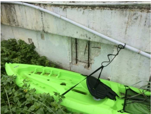
Large piece of concrete had fallen off seawall panel.
