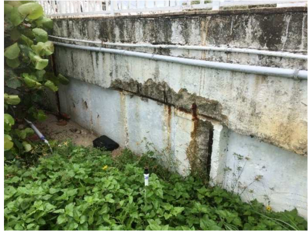
Severe corrosion damage and concrete spalling on both the seawall cap and panels
