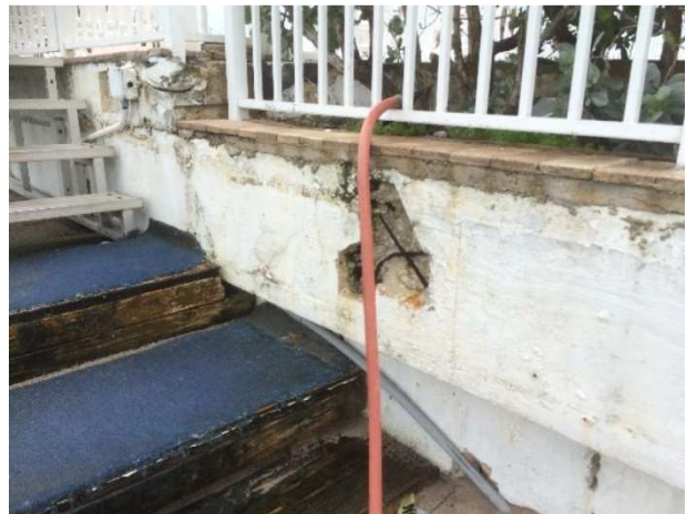
Concrete spalling on the seawall cap.
