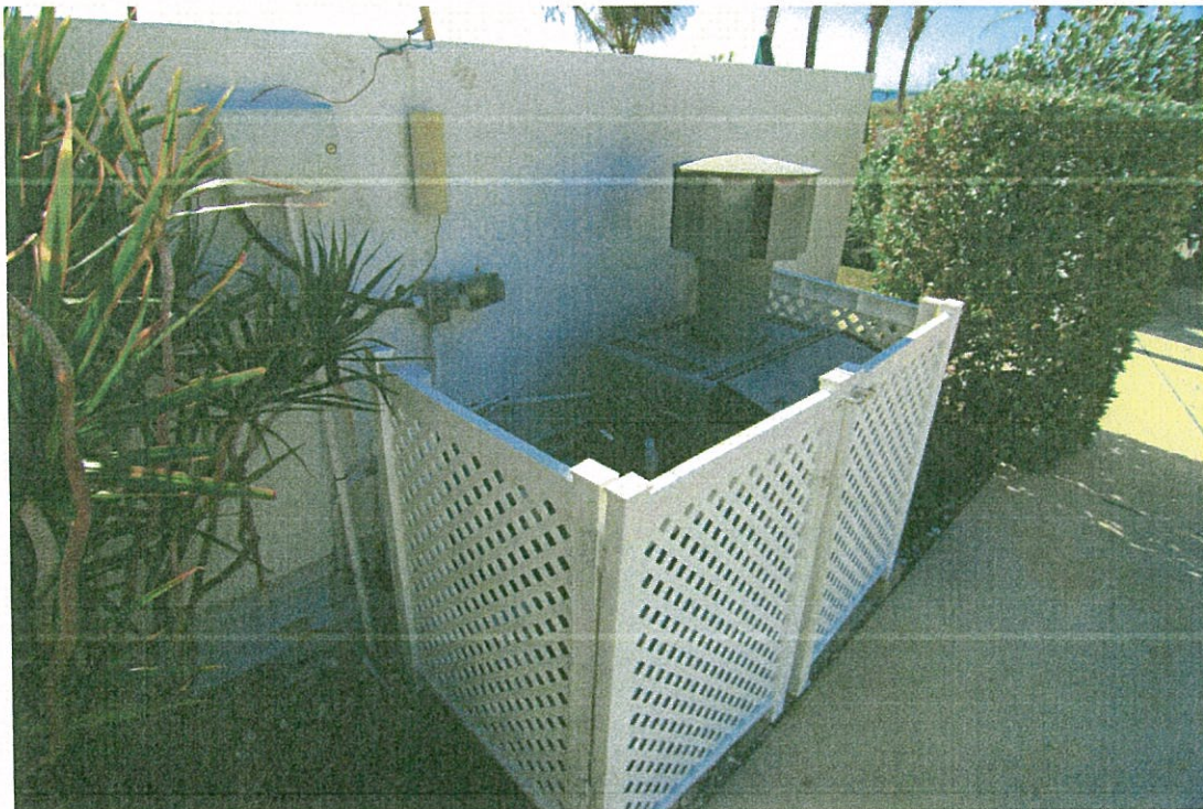
EXHIBIT 14. VIEW OF GAS HEATER, WEST SIDE OF POOL EQUIPMENT BUILDING
