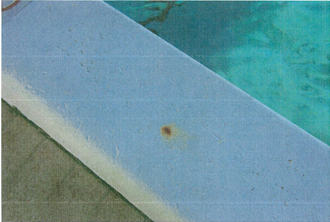
EXHIBIT 9. VIEW OF RUST STAIN ON COPING STONE
