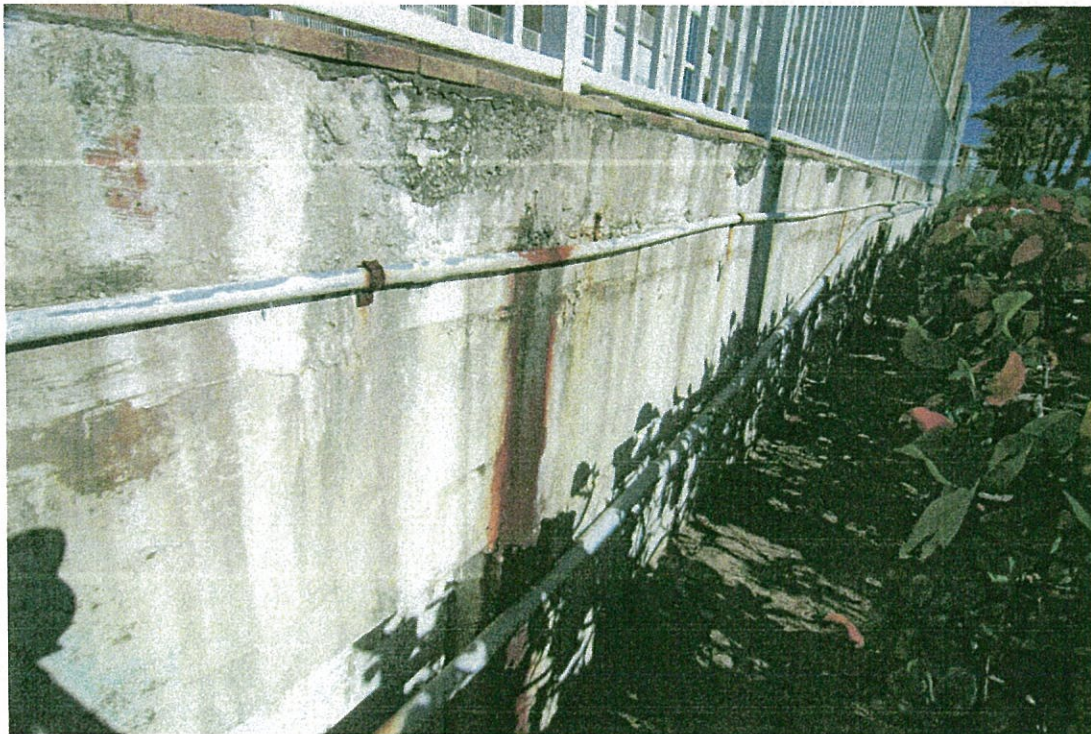
EXHIBIT 18. VIEW OF RUST STAINS ON RETAINING WALL, EAST SIDE OF POOL AND DECK
