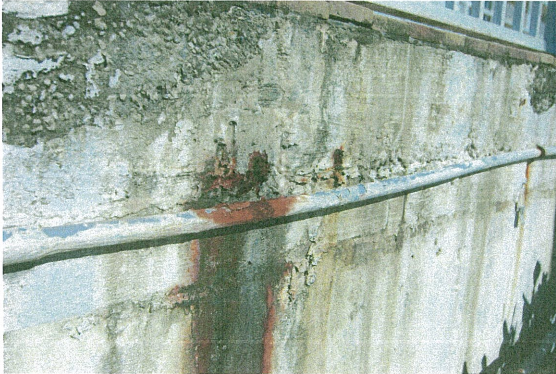
EXHIBIT 19. CLOSE-UP OF RUST STAIN FROM PIPE CLAMP ON RETAINING WALL, REFERENCE EXHIBIT 18
