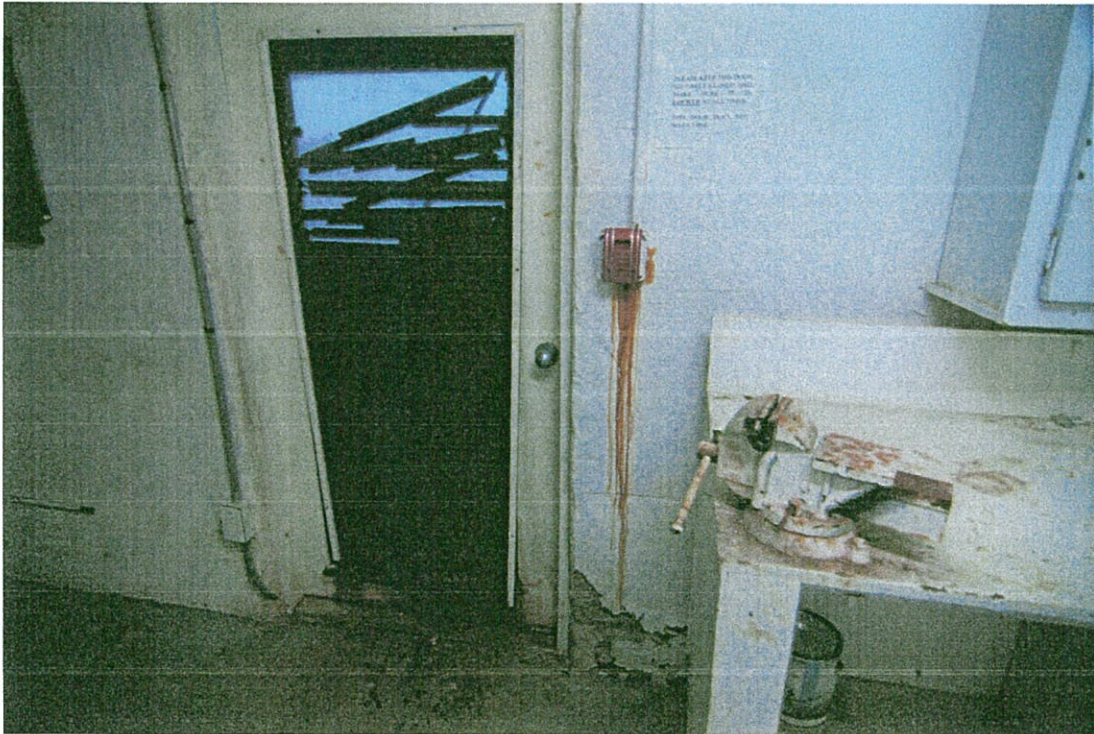
EXHIBIT 17. VIEW OF DETERIORATED PASS DOOR AND SPALLED CONCRETE, ENCLOSED AREA AT ENTRANCE TO PARKING GARAGE
