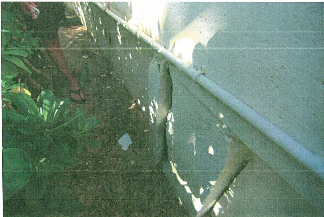
EXHIBIT 20. VIEW OF SPALLED CONCRETE ON RETAINING WALL, SOUTH OF BEACH ACCESS STEPS FROM POOL DECK
