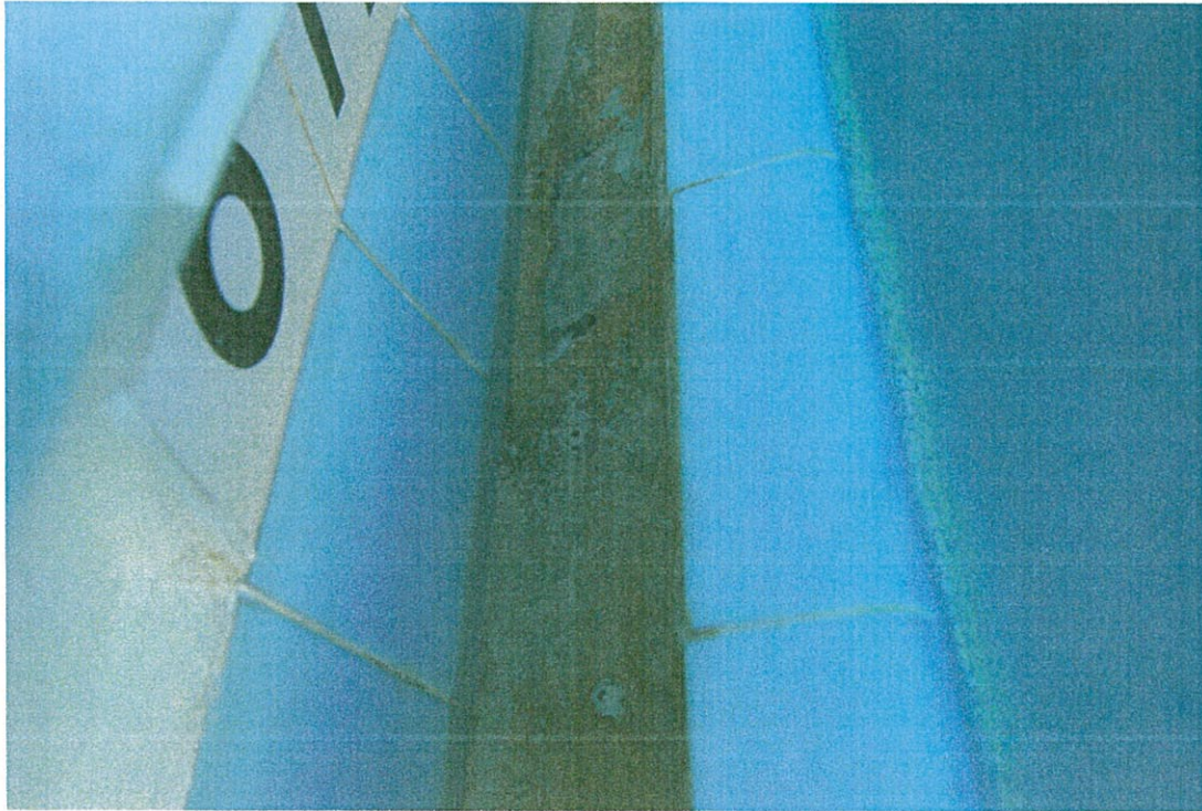
EXHIBIT 3. VIEW OF ERODED BEAM TROUGH FINISH
