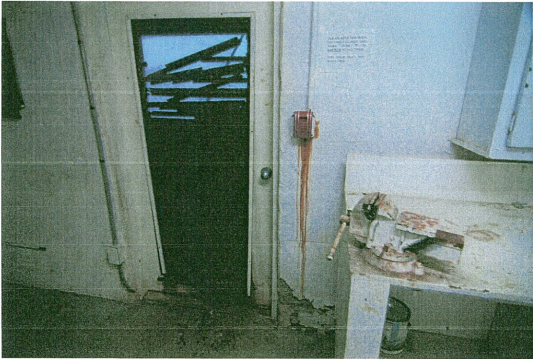
EXHIBIT 17. VIEW OF DETERIORATED PASS DOOR AND SPALLED CONCRETE, ENCLOSED AREA AT ENTRANCE TO PARKING GARAGE
